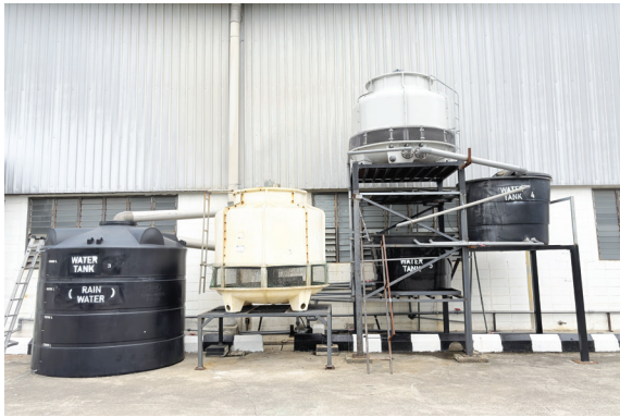
Cooling water system
